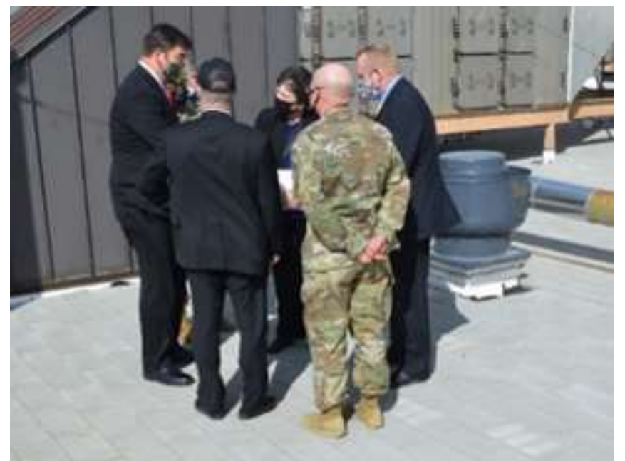
During her visit, ID-R Director Brenda McCullough (center), went to the rooftop of the Combined Chemical Test Facility (CCTF) to see the building's new roof. The CCTF supports the testing of protective clothing and masks, detectors and decontamination systems using chemical agents as challenge material. Getting a new roof for the 35,000-square-foot building was a top priority. Pictured here (clockwise from center) ID-R Director Brenda McCullough, Chemical Test Division Chief Dr. Chris Olson, DPG Commander Col. Scott Gould, Deputy Garrison Manager Chris Damour, Garrison Manager Aaron Goodman and Installation Command Sgt. Maj. Mauvet Rawls.
