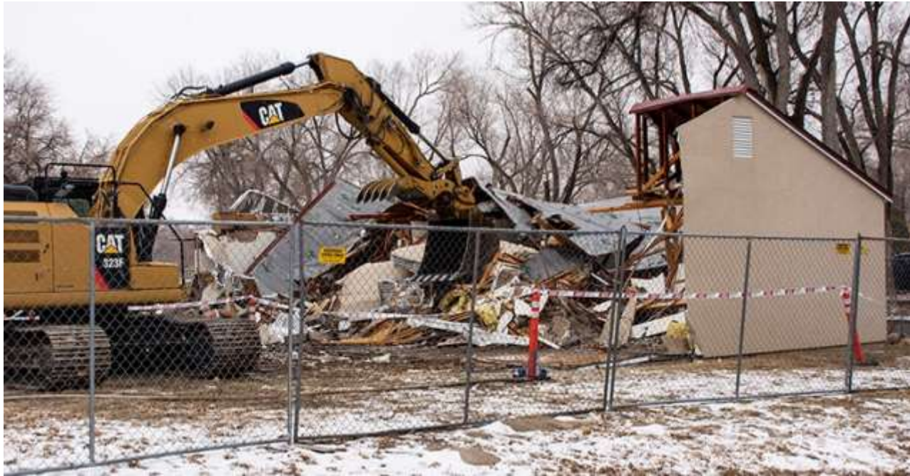
Heavy machinery takes down portions of the housing unit on 213 East Fifth, as one of 38 houses on East Wherry streets to be demolished. Built in the 1950s, the houses have become more expensive to maintain unoccupied than to demolish. Photo by Al Vogel, Dugway Public Affairs
