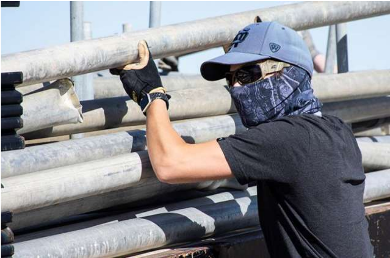
Christian Courtney stacks 3-inch aluminum pipe, left over from a test many years ago, onto the bed of a truck for recycling. Photos by Al Vogel, Dugway Public Affairs
